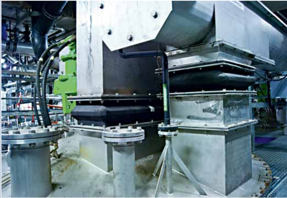
Elastomer expansion joints, type GU110 in the chute between the screw conveyor and sludge container in a slurry incineration facility NG 400 x 400, 60°C
