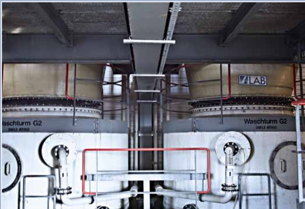
Elastomer expansion joints, type GU100 on the scrubbing drums of a waste incineration plant NB 2400, 80°C
